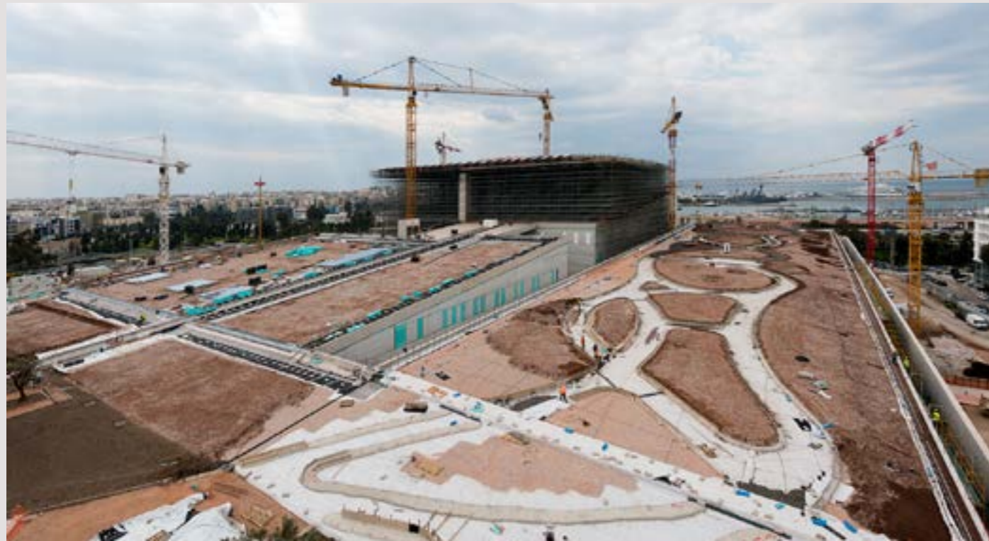
The SNFCC was dubbed the “triple project” since, in addition to the NLG and the GNO, it also included the creation of Stavros Niarchos Park.
